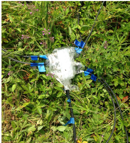
Figure 2-3 Infiniband cable box with eight channels plugged in. Plastic wrap is used to protect the connections from water and dirt. The experiment had four of these placed throughout the field.
