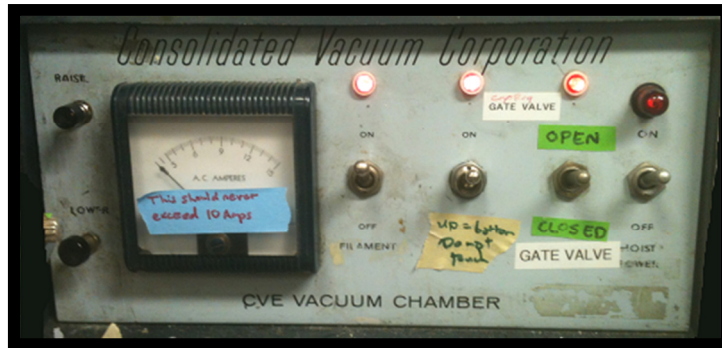
FIG B. CONTROL PANEL –
