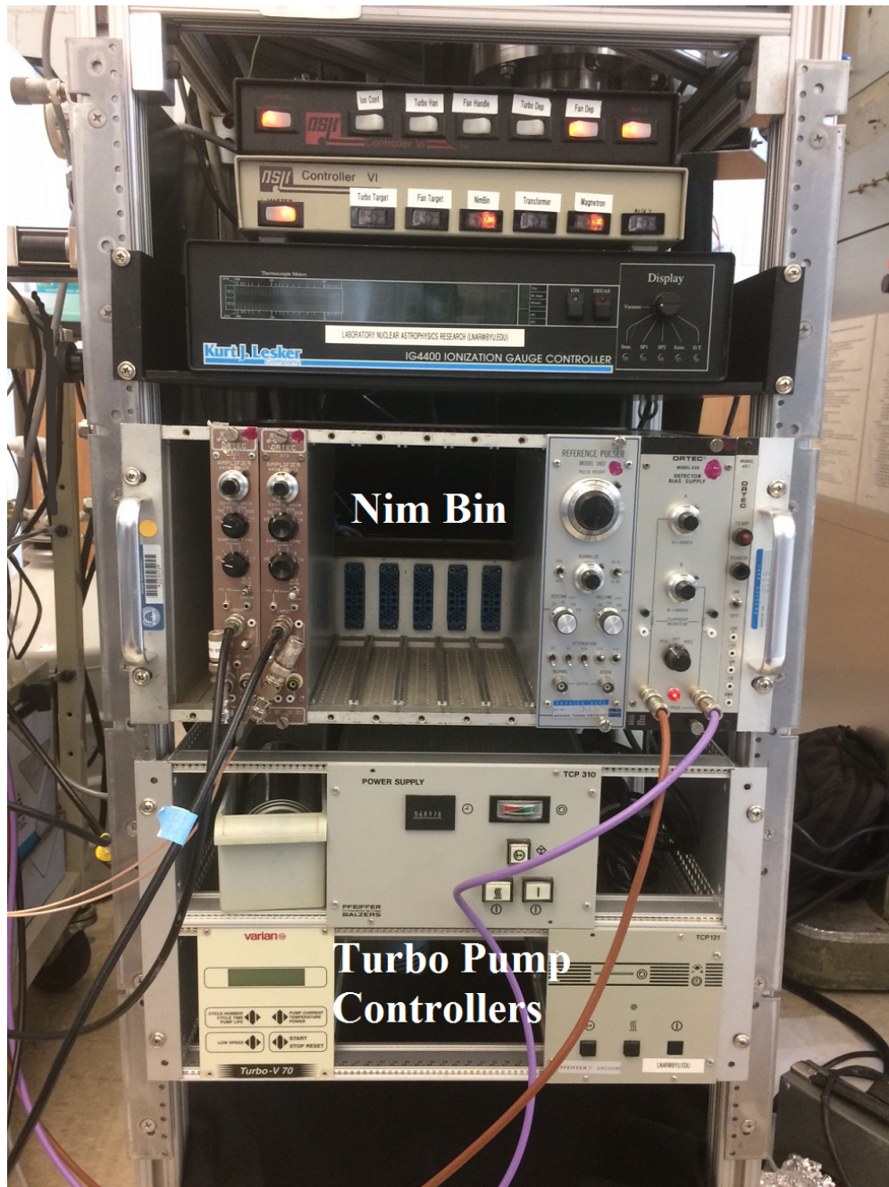
Figure 2.11 The top two bins are relays which power the everything on the system; it may be difficult to see but the switches are labeled according to what they power. Directly below them is the Ionization Gauge controller, which reads the pressure from the Ion gauge, as well as the thermocouples. The Nim Bin powers and amplifies the charged particle telescope described in 2.13. Lastly there are the three turbo pump controllers which power and monitor the speed of the turbo pumps.
