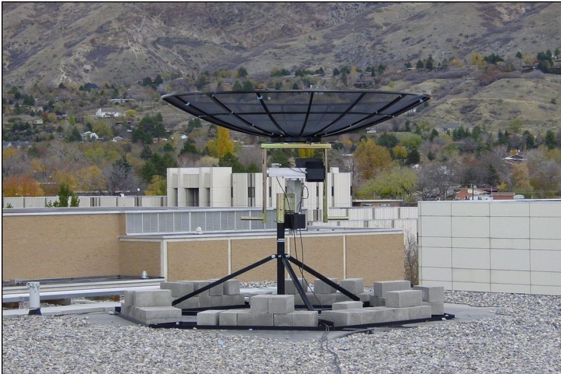
Figure 6-3: One of the VSA Antennas Located on The Engineering Clyde Building on the BYU Campus, shown with its mounting base, azimuth/elevation controller, counter weights, and base weights. Photo courtesy the BYU Electrical Engineering Research Group of Dr. Brian Jeffs and Dr. Karl Warnick.
