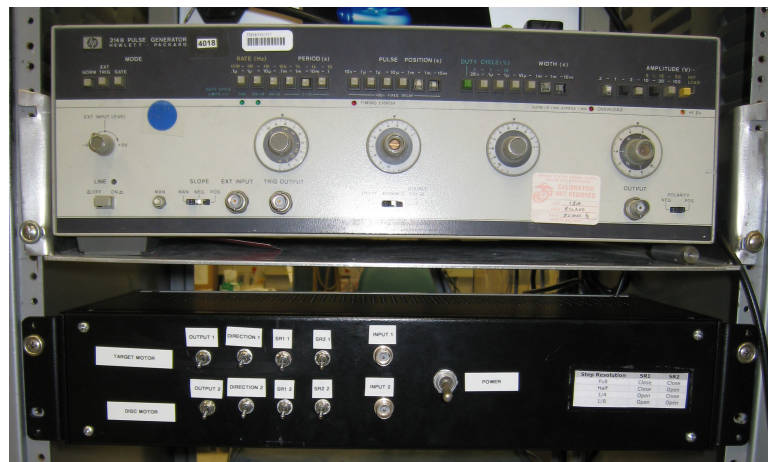
Figure 2.4 The control box is sitting below the HP Signal Generator
